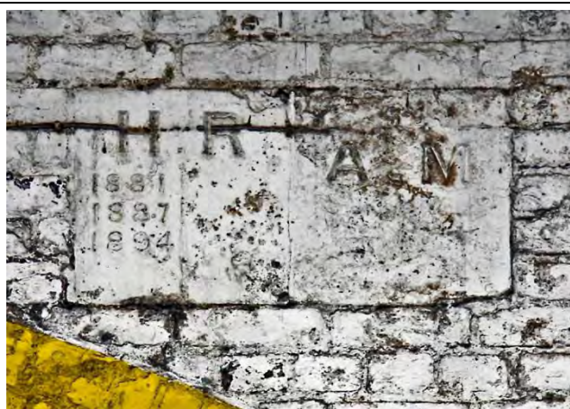
PBM 708. Yorkshire Road, E14, Fixed into railway viaduct immediately north of junction with Brunton Place, in Arch 366. The RH side is St Anne Middlesex (AM), the S at top smaller. There are traces of lettering beneath. LH side is Ratcliffe with perambulation dates. Parish of Ratcliffe (Hamlet) and St Anne Limehouse. TQ362812
