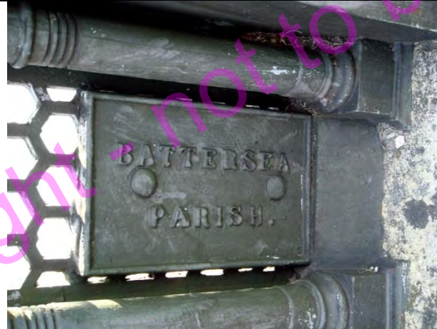
PBM 630. Battersea Bridge SW11, West side, near centre towards bottom of parapet. This mark (mounted on its end) is directly beneath PBM 403. Chelsea parish with Battersea parish. TQ269773
