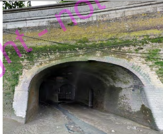
PBM 756. Chelsea Embankment, SW3. Foreshore, 280 yds west of Chelsea Bridge at base of parapet on river side above Ranelagh Sewer outfall. Image shows outlet tunnel. Boundary mark above outlet (on right hand side) at base of parapet.
