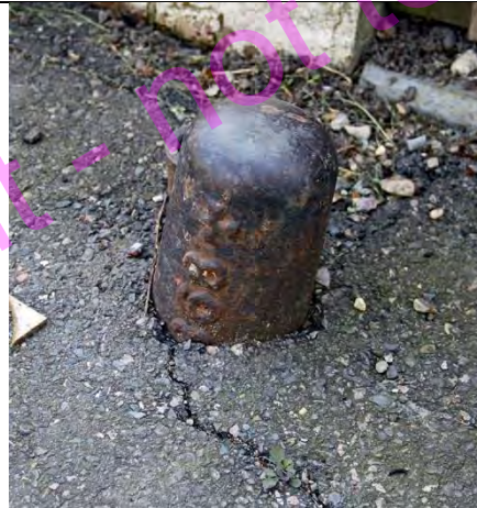
PBM 741. Kent House Road, SE26. West side by street name-board north side of entrance to Orchard Court (No 72 K.H.Rd). Remarkably this post has now virtually sunk out of sight. The cross suggests a Beckenham post and date 1868 is just visible. Parish of Beckenham with Lewisham. TQ3615771189
