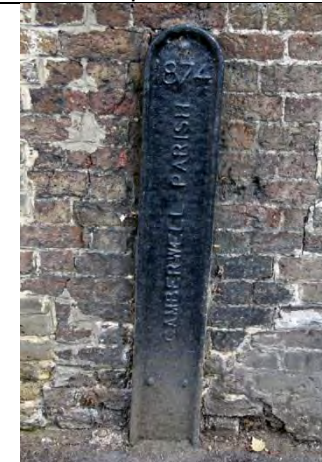
PBM 527A. Champion Hill SE5, Immediately to the right of PBM 527. This 4ft high mark, dated 1874, is similar to PBM 523.
